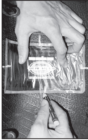
5. Centre the repair over the injury until the lines on the liner and the lines on the are coinciding. Mark the area around the repair with chalk.
