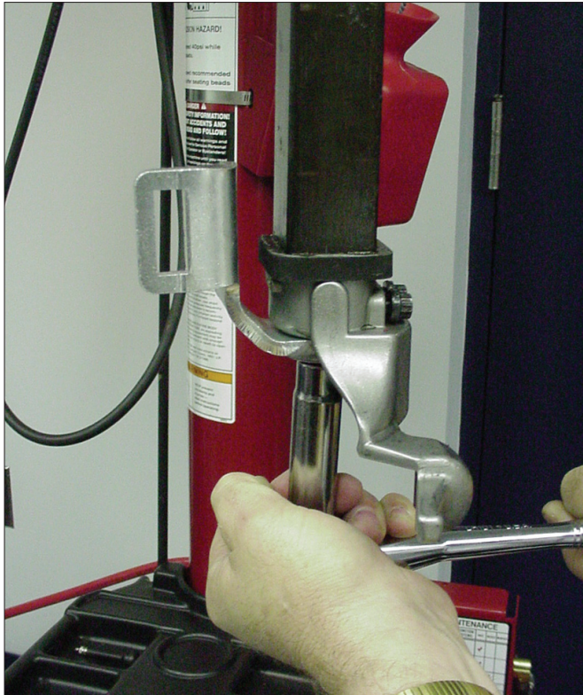
Figure 17 - Install bracket to the vertical slide.
